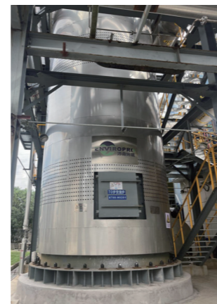
Waste Gas Incinerator
